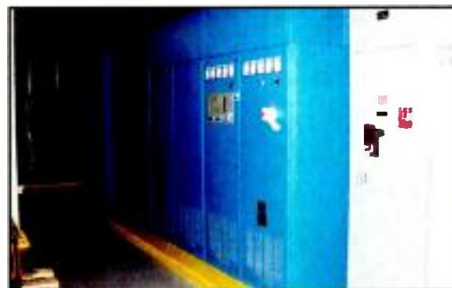
A facility-wide UPS system needn't power everything. Focus first on critical on-air and playout systems that may fail with even a millisecond interruption in power.
